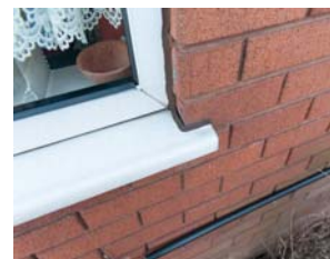
Failed silicon sealant identified and recorded on survey
